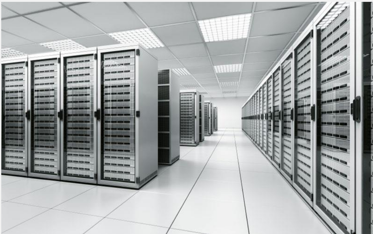
Stock image © https://commons.wikimedia.org/wiki/File:Img_51614_critical-data-centre-at-uni-of-hertfordshire.jpeg
